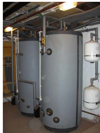
2 x 300l VPA hot water cylinders
